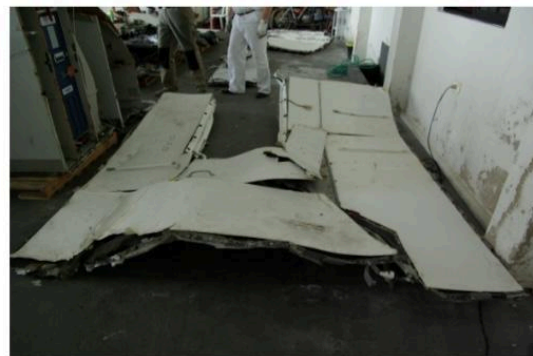
Figure 39: Ceiling of the LDMCR: with top-downwards deformation
